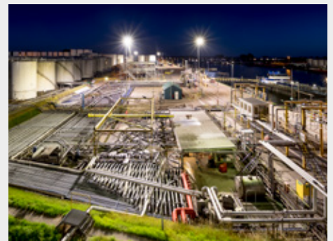
Tank storage Standic B.V. | Dordrecht | Netherlands
